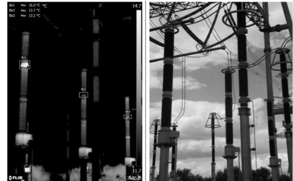
图5 500 kV 电容式电压互感器三相红外热像图 Fig. 5 Three-phase infrared thermogram of 500 kV capacitor voltage transformer
