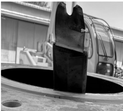
图 10 联接片破损脱落 Fig. 10 Damage and fall-off of connection piece
